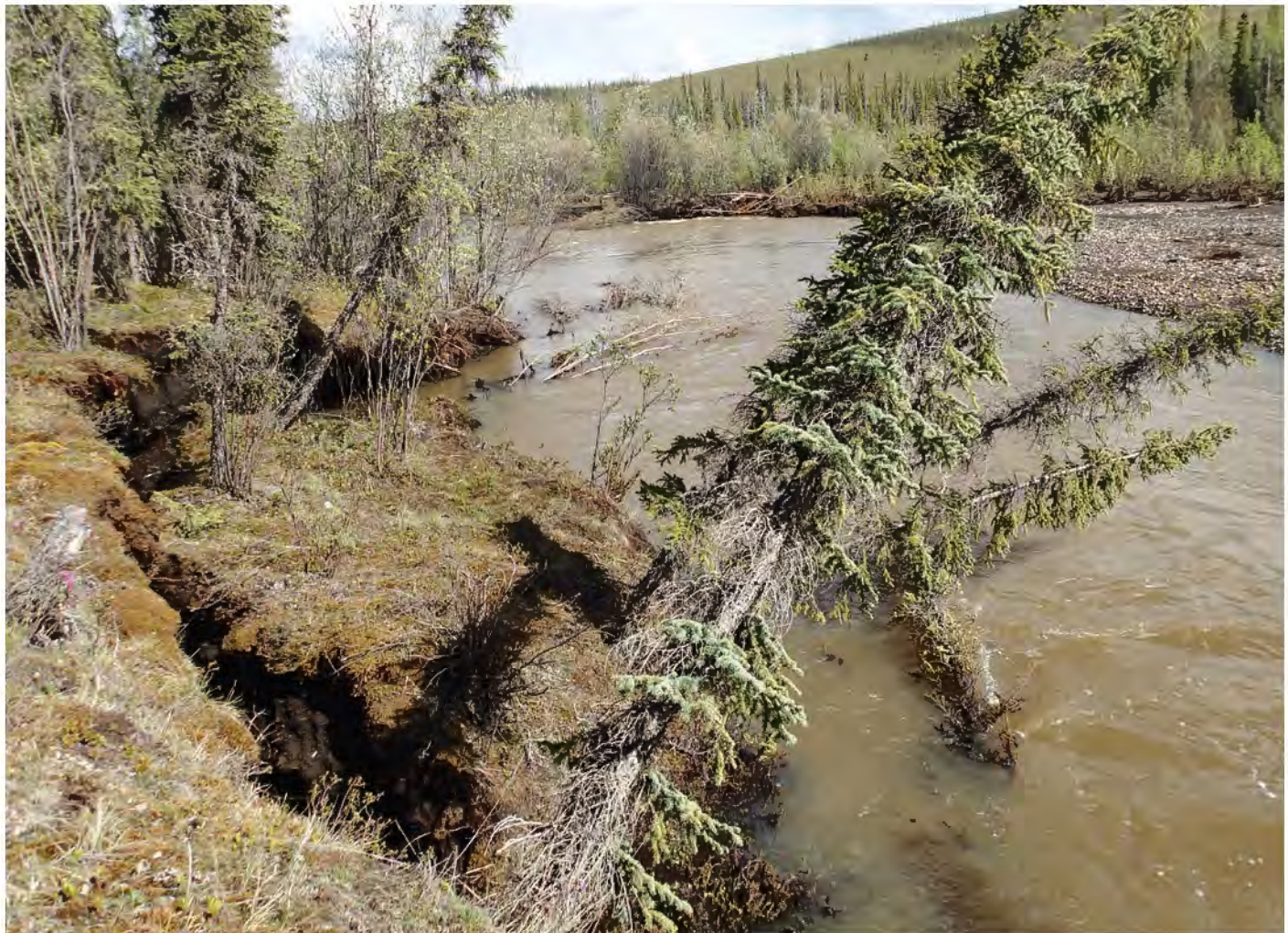
Collapse of undercut riverbank due to thawing and erosion of permafrost by high flows along Engineer Creek, Yukon
